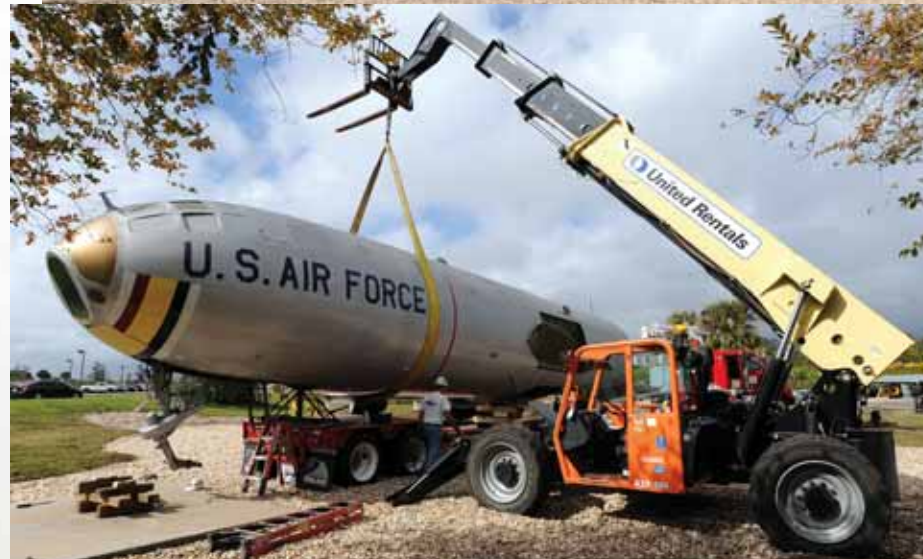
Corroded hardware and fasteners made the disassembly of the four-engine Cold War warrior difficult. On 10 January, the fuselage was being secured to a lo-boy trailer.
